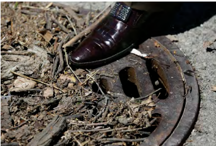
FIGURE RR-5: Aging and Limited Infrastructure
