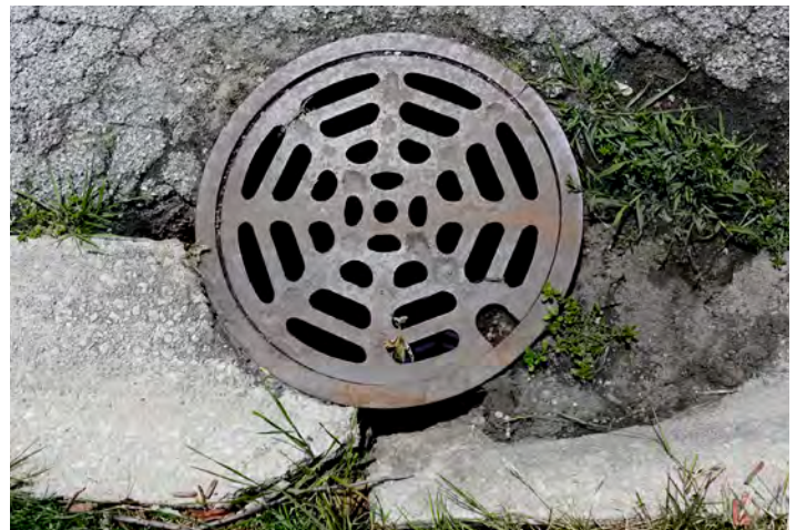
FIGURE RR-6: Degraded Sewers
