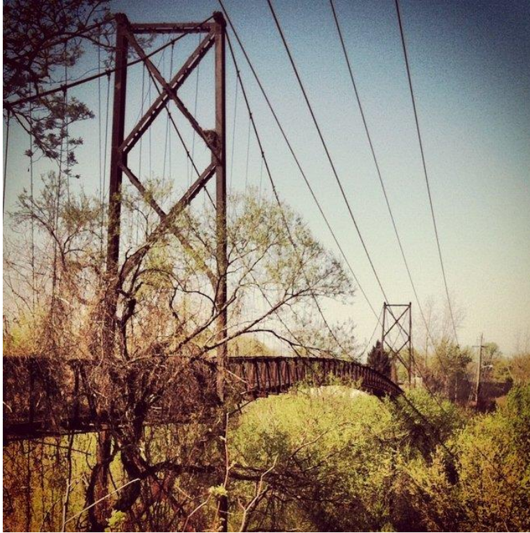
Figure 8 The Sidaway Bridge once provided a pedestrian for the neighborhood, but has been closed for decades. Image Source: Matthew Ciampini, Sidaway Bridge, Cleveland.com Photo Gallery.
