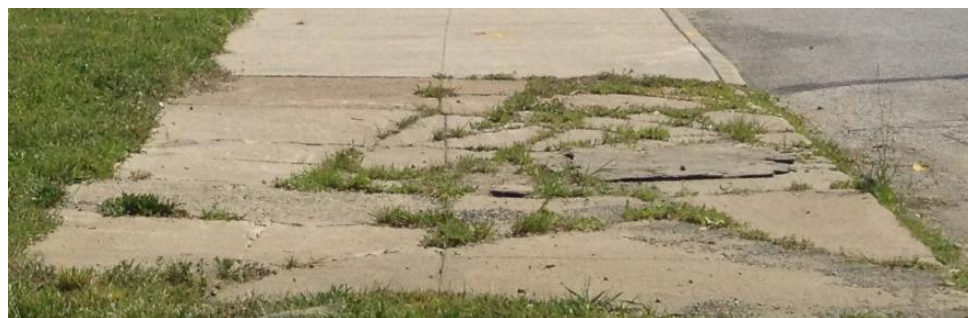
Figure 7 Dilapidated sidewalks in some parts of the neighborhood could be improved to make walking more appealing.
